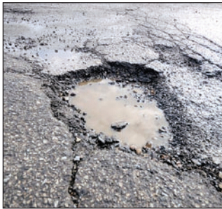
pothole on a street
